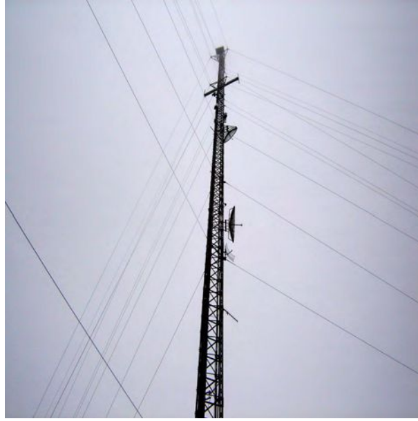
Figure 1: Typical guyed tower for mobile signal transmission.
