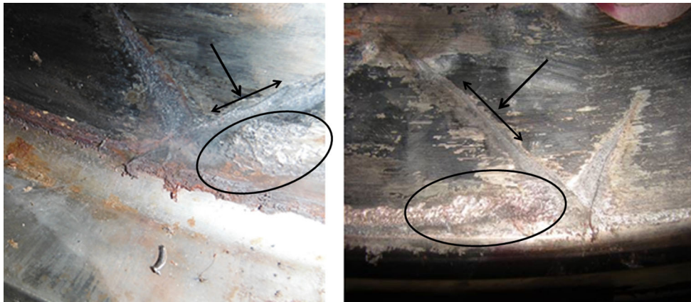
Fig. 4 Cracking of shaft (left) and coupling (right) before opening fracture surfaces. Cracking is pointed out in arrows (with the main fracture plane indicated in black) and fretting damage circled
