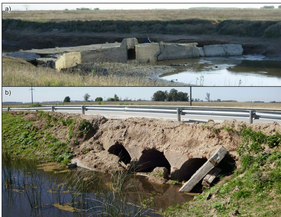
Fig. 3 State of bridges and culverts in different sections of the basin. a abandoned bridge in sector G, close to Veronica town, b obstructed culverts in PR 6, sector A (see Fig. 2)
