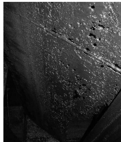
Fig. (5). Photograph showing filter with attack (pitting).
