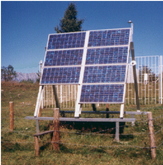
Fig. 3a PV-Powered Pollution Control Unit
