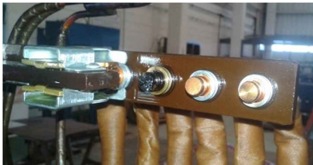
(a) Case 1: high resistance point on the fixed contact of the De-energized tap changer (DETC).
