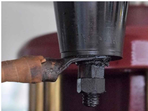
(c) Case 4: loose bushing contact inside the tank.
