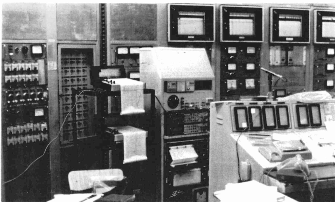
Fig. C.1.3: Panel de control.
