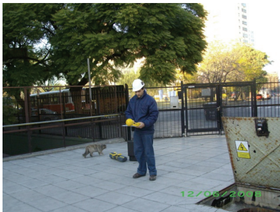
Figure 12: Measurement in a Distribution Substation (CT32)
