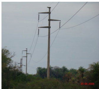
Figure 5: Power Line 132 kV (LA24)
