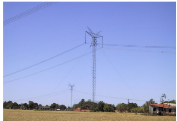
Figure 2 - HVDC Tower 600 Kv
