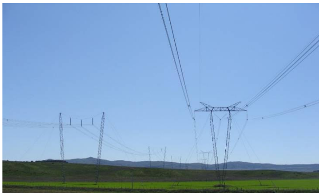
Figure 1 - HVAC Towers 500 kV
