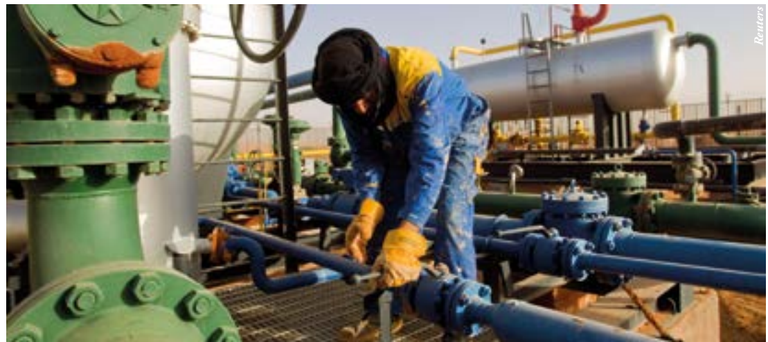
A worker is seen at the Zarzaitine gas field in In Amenas, southeast of Algiers.
