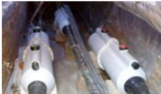
Passive loops HV Cable Joints
