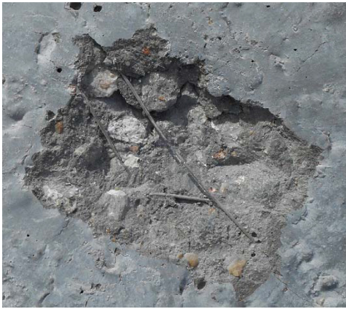
Fig. 15. Eroded zone of slab F801.
