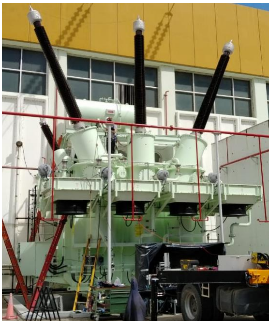
Fig. 5. Caso 3: 353/13.8 kV – 140 MVA
