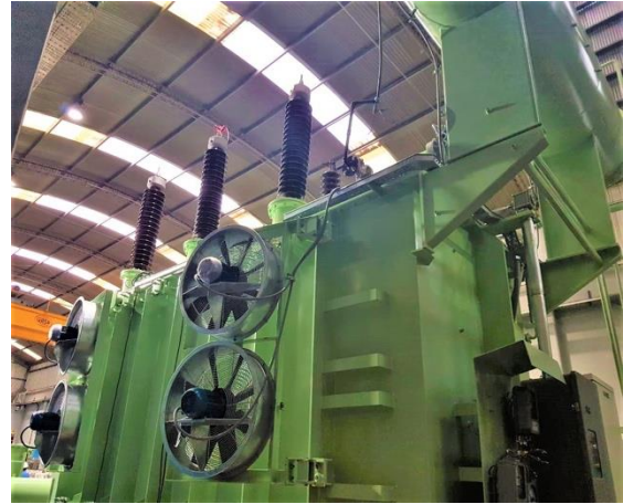
Fig. 4. Caso 2: 132/34.5/13.8 kV – 40 MVA – YNyn0d11
